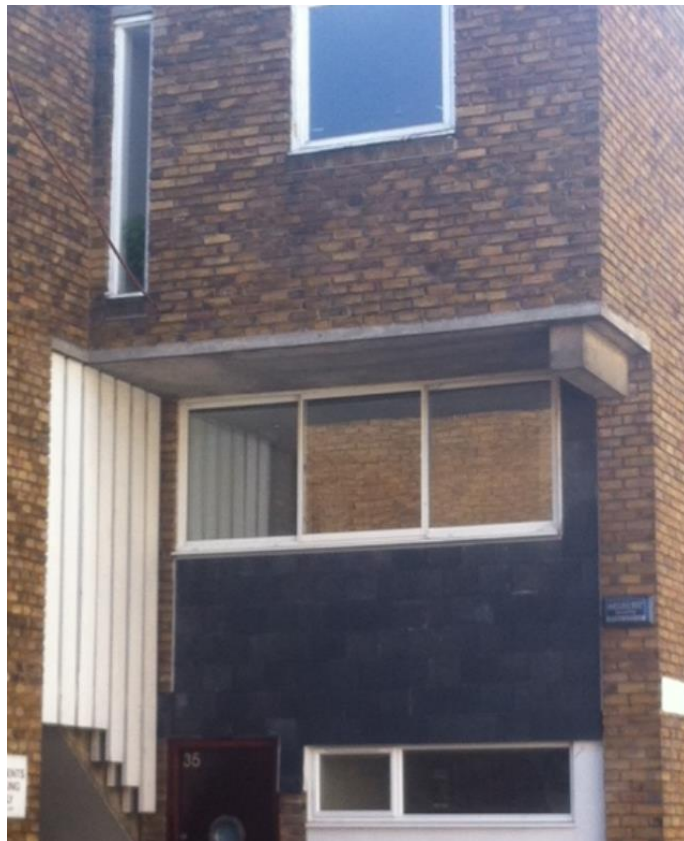
Image 6: Existing variation to window frames in Legion Close with Aluminium, Timber and UPVC
